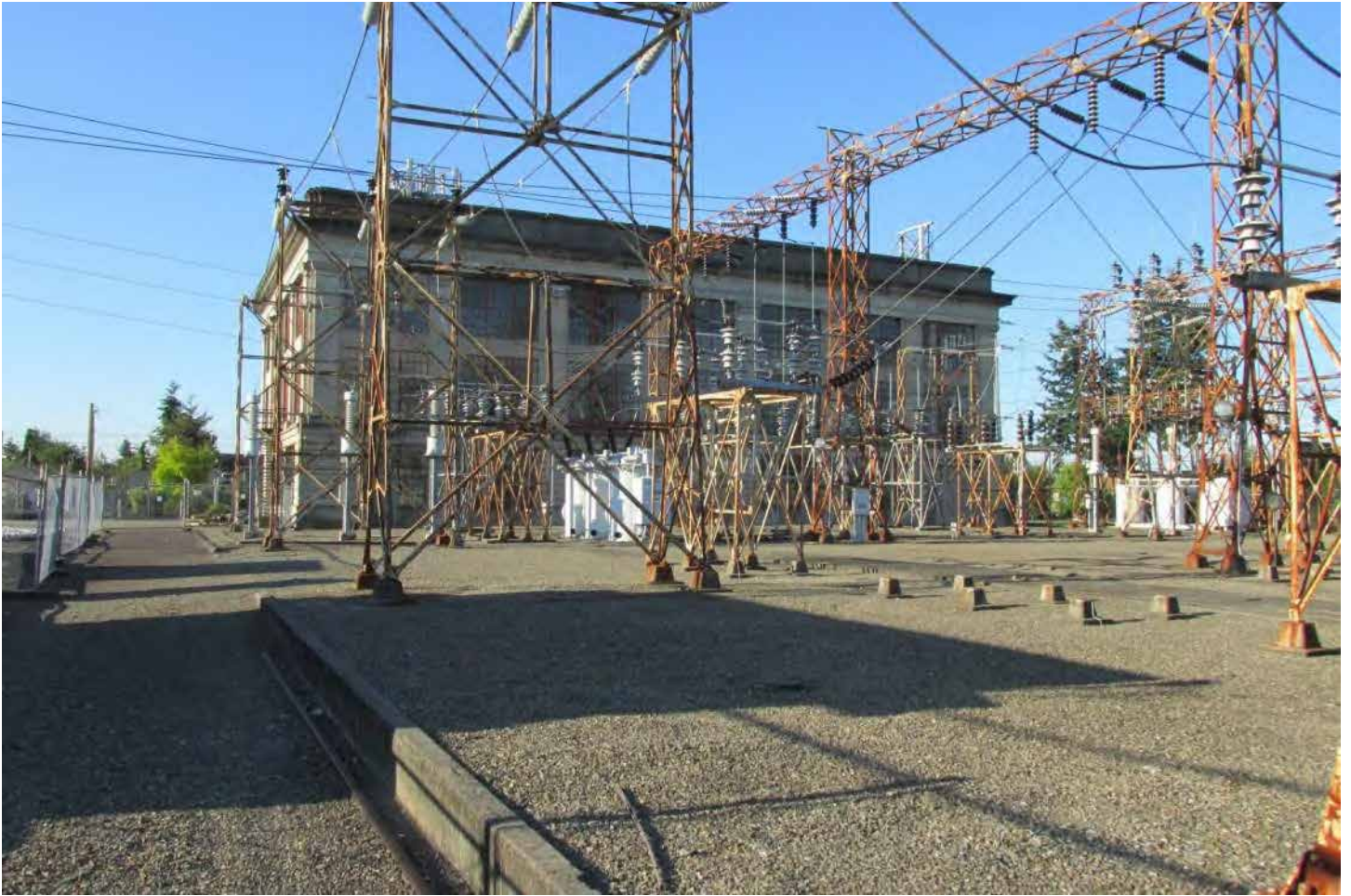
Figure 20 Cushman Substation view south
