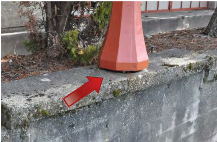
There is a gap under some lamp posts. Image by Richaven Architecture and Preservation.
