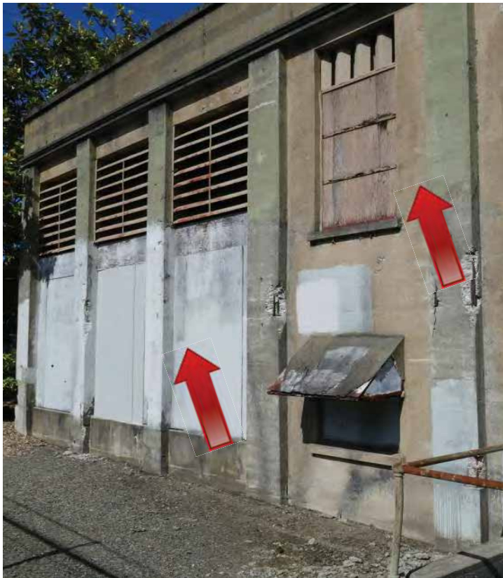
Missing windows and openings for ventilation under the louvers have been covered with plywood boards. Historical photos show single steel-framed nine-light windows with louvered vents above. Image by Richaven Architecture and Preservation. 220620 CoT CAS EL-W P1000685.JPG
