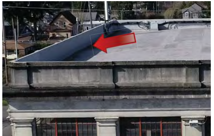
The back of the parapet on the south elevation has algae, indicating that water is collecting. Image by Richaven Architecture and Preservation. 200224 CoT CAS EL-E DJI_0006.JPG
