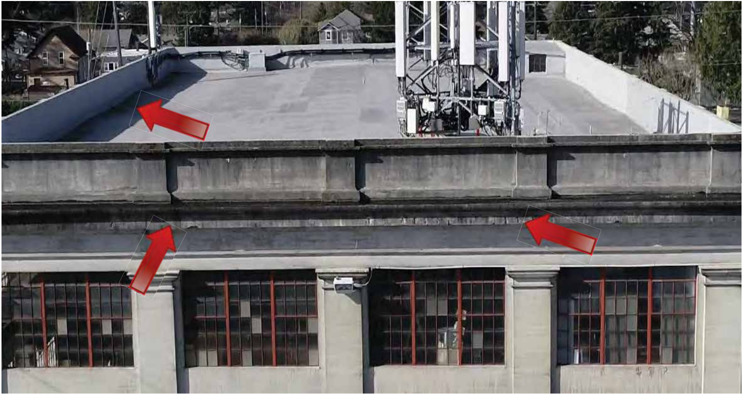
The back of the parapet on the south elevation has algae, indicating that water is collecting. There is also severe spalling on the cornice on the east elevation. There is a significant amount of atmospheric soiling. Image by Richaven Architecture and Preservation. 200224 CoT CAS EL-E DJI_0006.PNG
