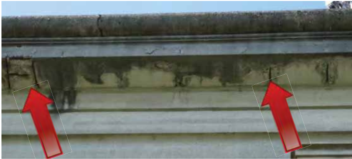
Exposed reinforcing steel and spalling under the cornice on the west elevation. Image by Richaven Architecture and Preservation. 220620 CoT CAS EL-W P1000666.JPG
