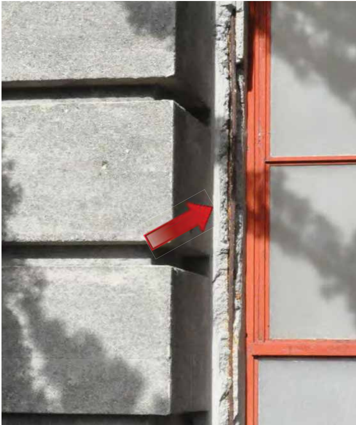
Spalling around a window frame on the west elevation and reinforcing steel bar exposed due to carbonation-induced corrosion. Often occurs in areas with a shallow concrete cove Image by Richaven Architecture and Preservation. 200224 CoT CAS EL-W DSC_0026.JPG
