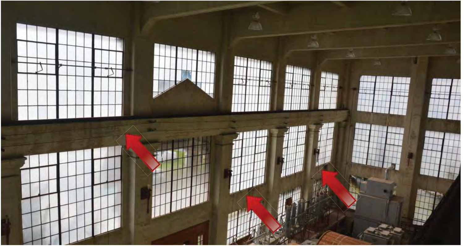
The dark areas under the windows appear to be organic growth (algae), indicating water infiltration. There is also a substantial amount of paint failure on the walls. Image by Otak. 200224 CoT CAS EL-INT DSC_0998.jpg
