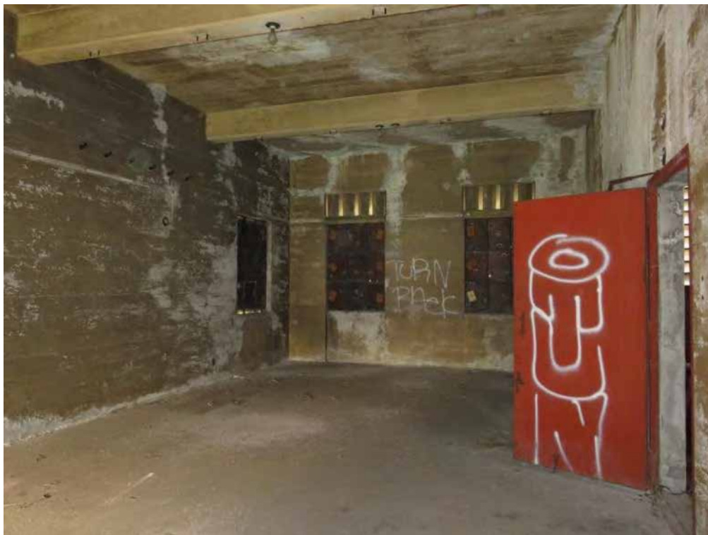
Photo 10 of 13. WA_PierceCounty_AdamsSt.Substation_0010. Adams St. Substation, interior, switch room, upper level, view west.
