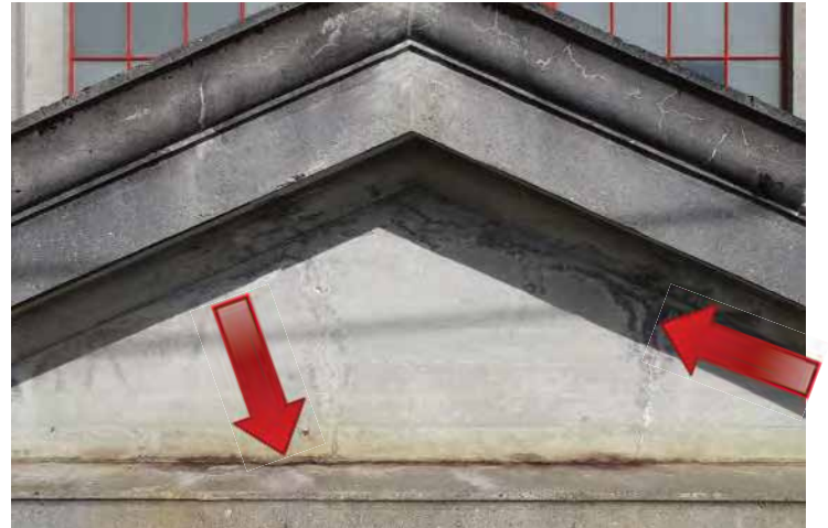
The pediment above the main entrance on the south elevation shows the build-up of atmospheric soiling that has adhered to the concrete and visible stains due to corrosion of the reinforcing steel. Efflorescence is also observed. Image by Richaven Architecture and Preservation. 200224 CoT CAS EL-S DJI_0023.JPG
