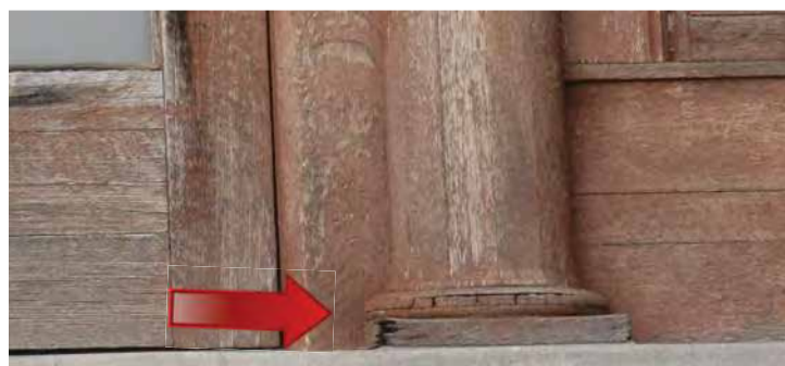
Some areas in the wood are severely rotted. Image by Richaven Architecture and Preservation. 200224 CoT CAS EL-S DSC_1063.JPG
