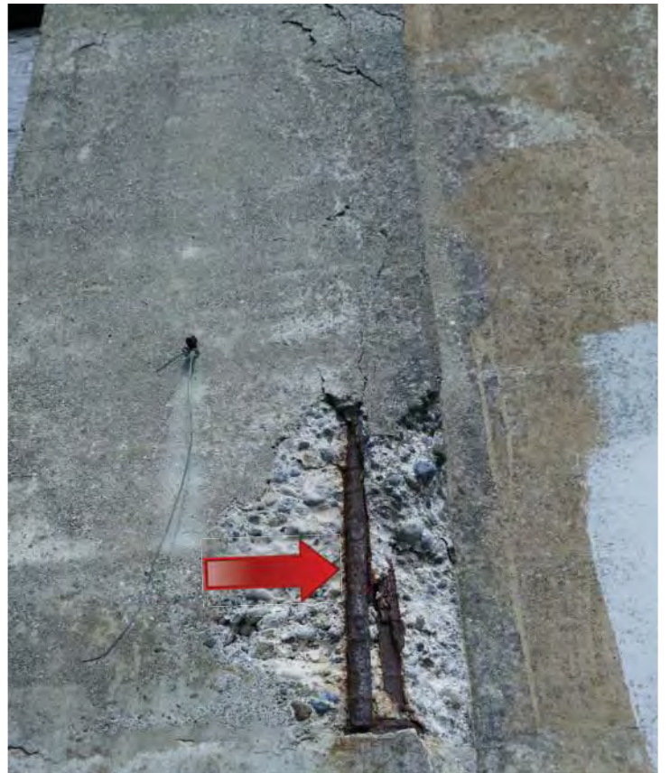
Severe separation from the substrate. Image by Richaven Architecture and Preservation. 220620 CoT CAS EL-W P1000679.JPG
