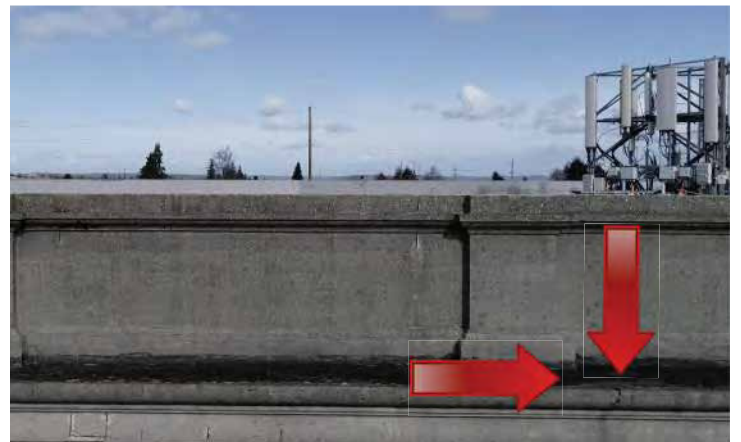
Water proofing on top of cornice appears to be failing. Image by Richaven Architecture and Preservation. 200224 CoT CAS EL-S DJI_0022.PNG
