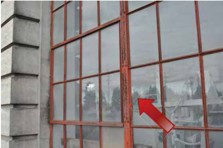
Steel with signs of corrosion. Image by Richaven Architecture and Preservation. 200224 CoT CAS EL-N DSC_0175.JPG
