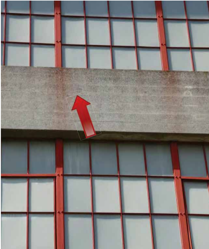
Bleeding marks of rust and paint have stained the concrete surfaces on all elevations of the building. Image by Richaven Architecture and Preservation. 220620 CoT CAS EL-W P1000667.JPG
