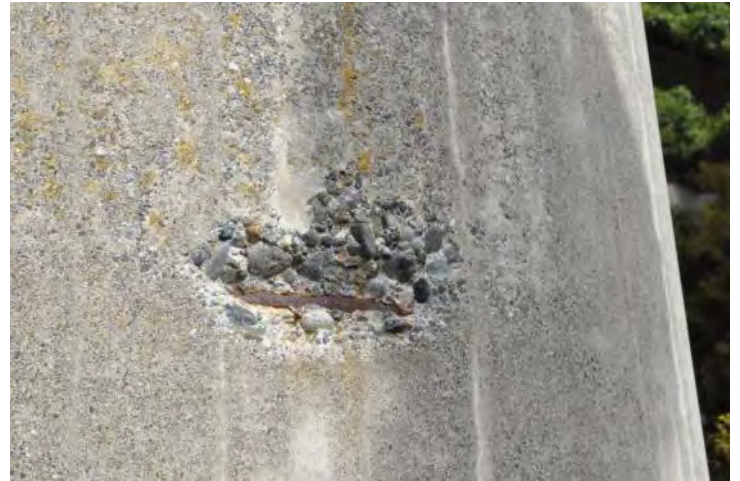
Reinforcing steel and aggregates being exposed on a wall corner on the west elevation. Spalling is present in all elevations on the building. Image by Richaven Architecture and Preservation. 200224 CoT CAS EL-S DSC_0013.JPG
