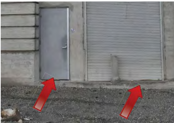
Doors on the north elevation are beginning to deteriorate. Image by Richaven Architecture and Preservation. 200224 CoT CAS EL-S DSC_0189.JPG
