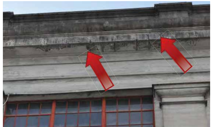
Spalling, efflorescence and atmospheric soiling under the cornice and capitals. Image by Richaven Architecture and Preservation. 200224 CoT CAS EL-N DSC_0163.JPG
