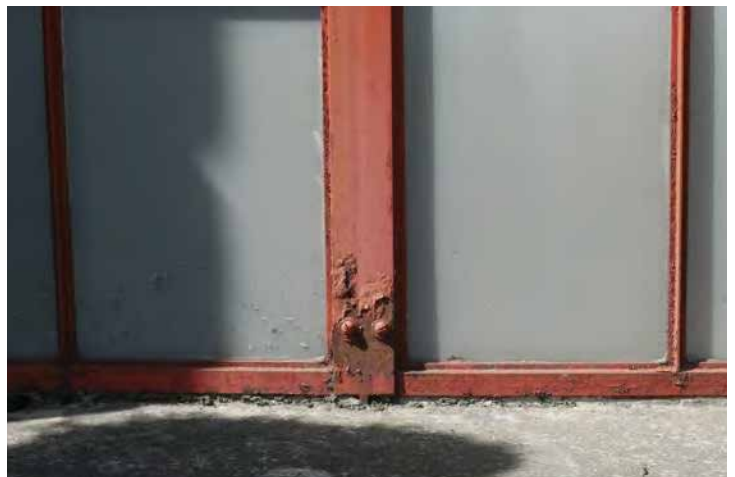
Visible corrosion around the fasteners of a window on the west elevation. Image by Richaven Architecture and Preservation. CoT CAS EL-W P1000654
