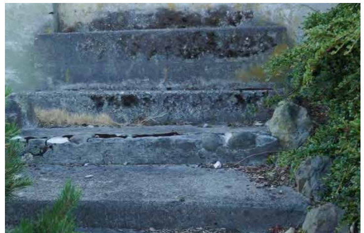
Organic soiling (algae and plants), observed on concrete stairs on the east elevation of the building. Image by Richaven Architecture and Preservation. 220620 CoT CAS EL-E P1000689.JPG
