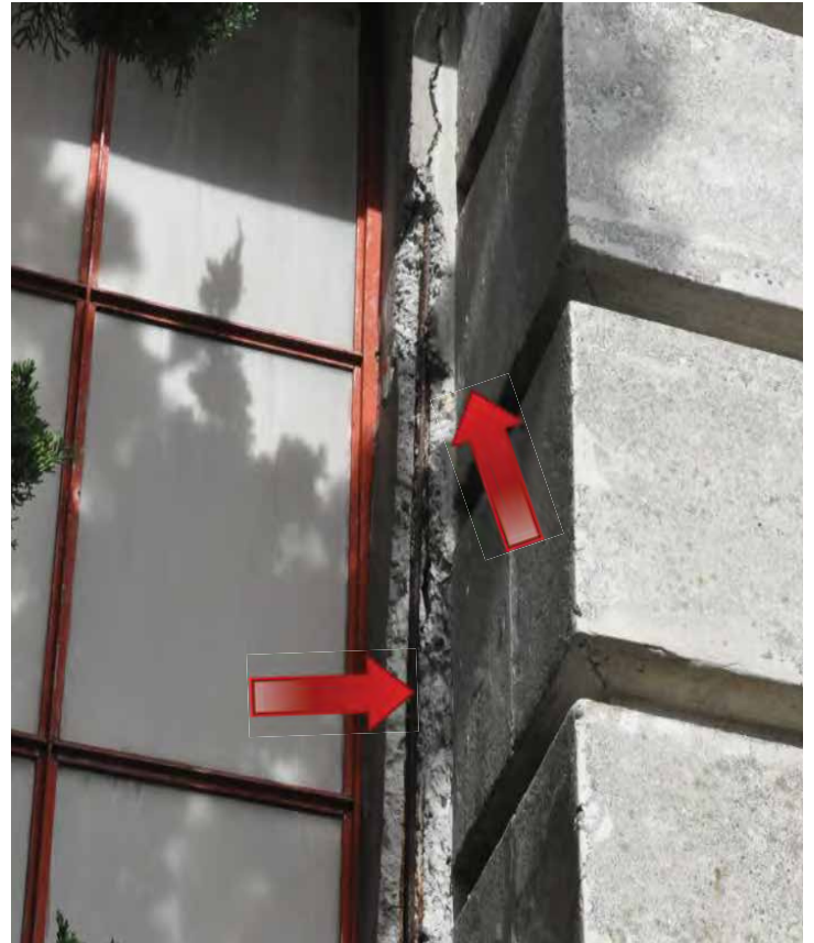
Exposed reinforcing steel and failed concrete around one of the ground-level window bays on the west elevation. There is some amount of corrosion visible. Image by Richaven Architecture and Preservation. 200224 CoT CAS EL-W DSC_0028.JPG
