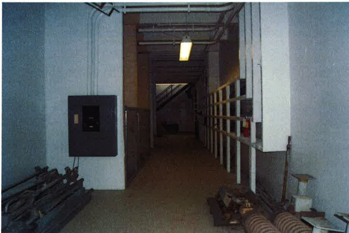
Photo 15 of 17. WA_PierceCounty_CushmanSubstation_0015. Basement level of Cushman Substation.
