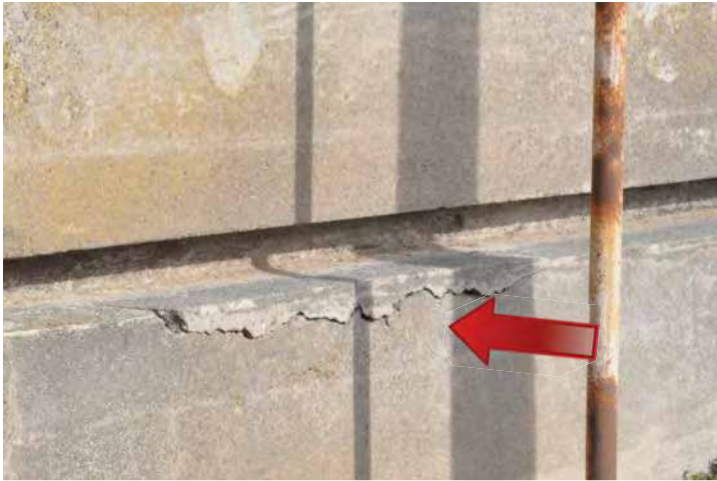
Cracks on the foundation, on the east corner of the south elevation. Image by Richaven Architecture and Preservation. 200224 CoT CAS EL-S DSC_0004.JPG
