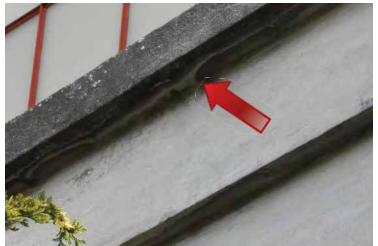
Efflorescence under a window ledge on the west elevation. Moisture infiltration will result in spalling. Image by Richaven Architecture and Preservation. 200224 CoT CAS EL-W DSC_0034
