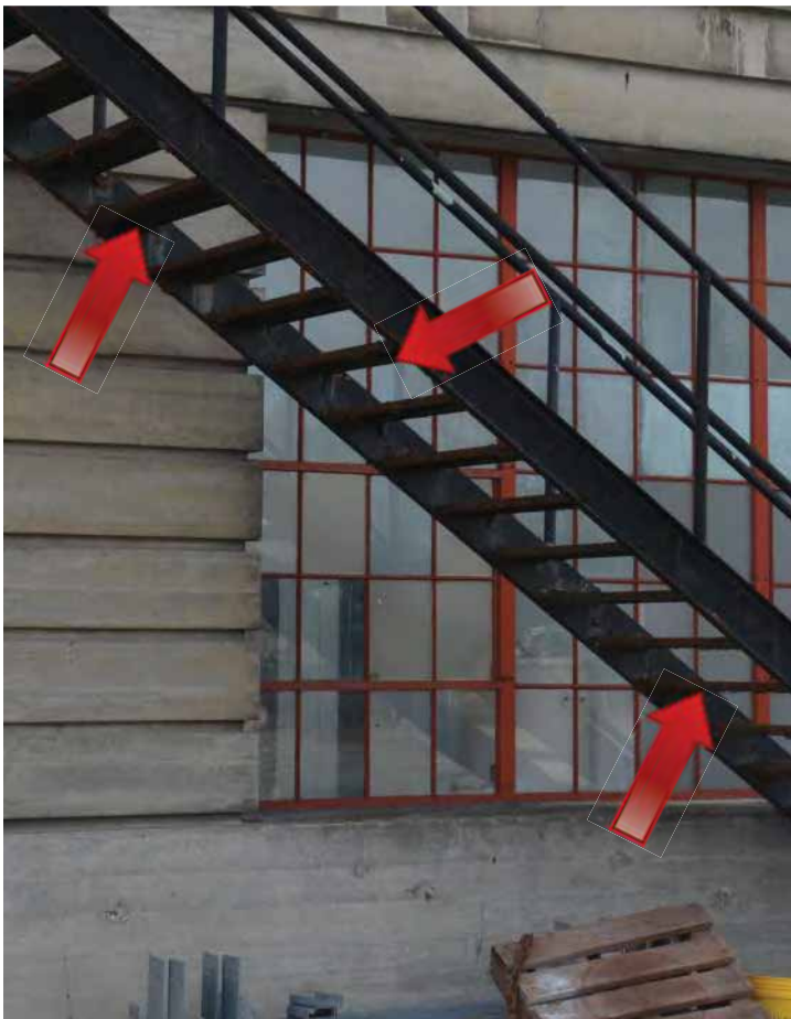
Richaven observed a substantial amount of corrosion on the steps and railings of the stairwell structure. Image by Otak. 200224 CoT CAS EL-E DSC_1045.JPG
