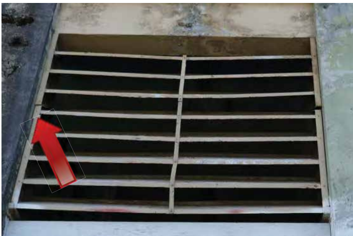
Metal louvers on the east elevation are bent and failing. There are visible gaps between the metal frame. Image by Richaven Architecture and Preservation. 220620 CoT CAS EL-E P1000692.JPG
