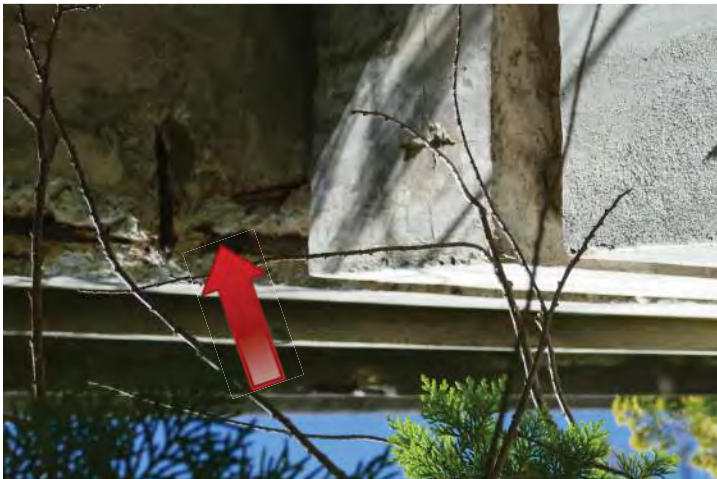
Looking up at the failed concrete at the upper left corner at a ground-level window bay, west elevation. The image below shows concrete debris that has separated from the substrate. Image by RichavenArchitectureandPreservation.220620CoTCASEL-WP1000663.JPG
