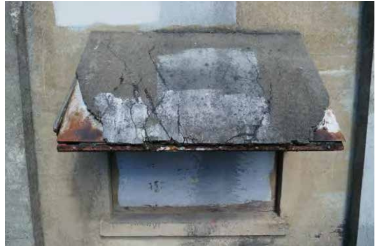
The metal awning on the west elevation is corroded. A layer of asphaltic material attached to its surface is severely damaged. Image by Richaven Architecture and Preservation. 220620 CoT CAS EL-W P1000680.JPG
