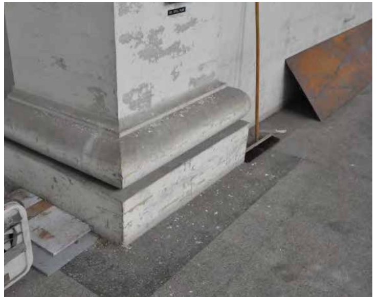
Paint failure and dust / dirt soiling on the base of the pilaster. Image by Otak. 200224 CoT CAS EL-INT DSC_0078.JPG
