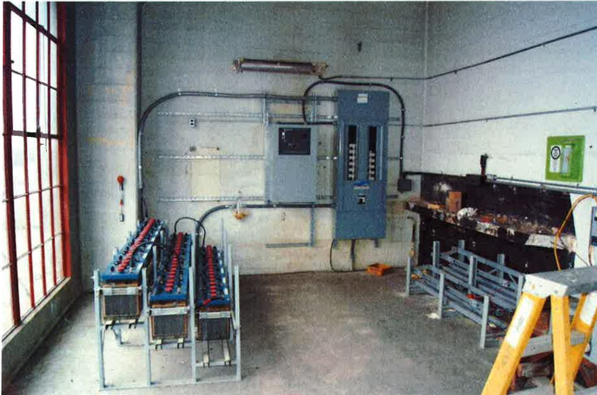
Photo 13 of 17. WA_PierceCounty_CushmanSubstation_0013. Battery room at Cushman Substation.
