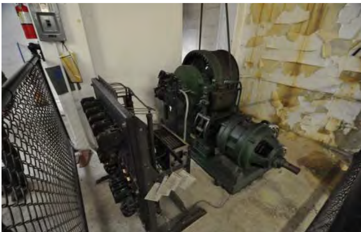
Paint failure, peeling, and soiling on walls. Image by Otak. 200224 CoT CAS EL-INT DSC_0125.JPG
