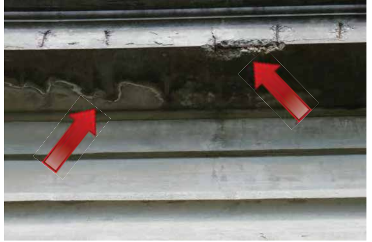
Section of the cornice on the west elevation shows spalling and reinforcing steel exposed due to water infiltration. Image by Richaven Architecture and Preservation. 220620 CoT CAS EL-W P1000649.JPG
