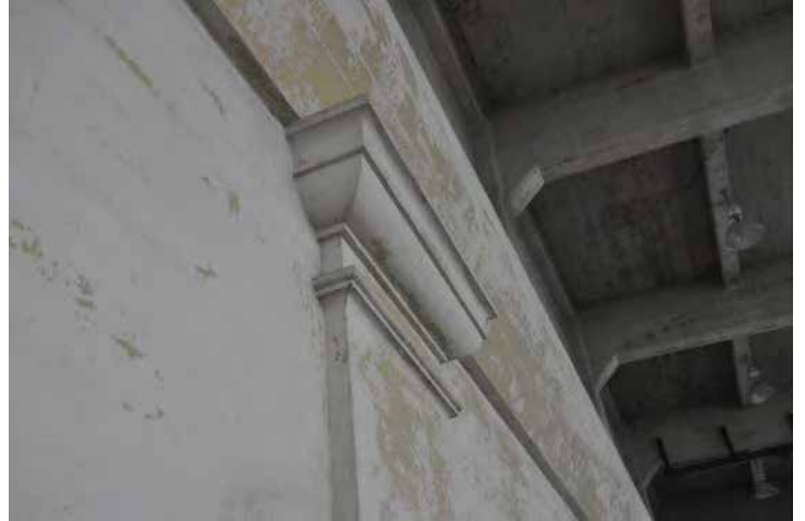
Visible paint failure, flaking, and peeling. Image by Otak. 200224 CoT CAS EL-INT DSC_0082.JPG.
