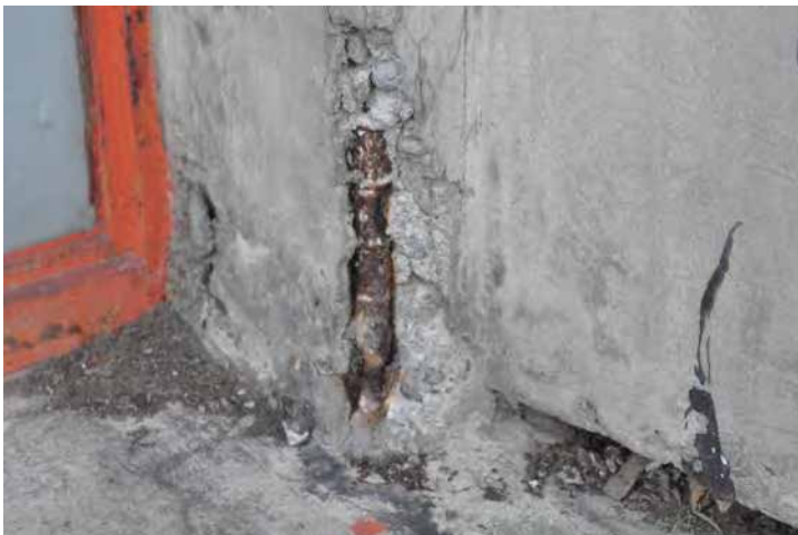
Exposed reinforcing steel with corrosion. Image by Richaven Architecture and Preservation. 200224 CoT CAS EL-N DSC_0174.JPG
