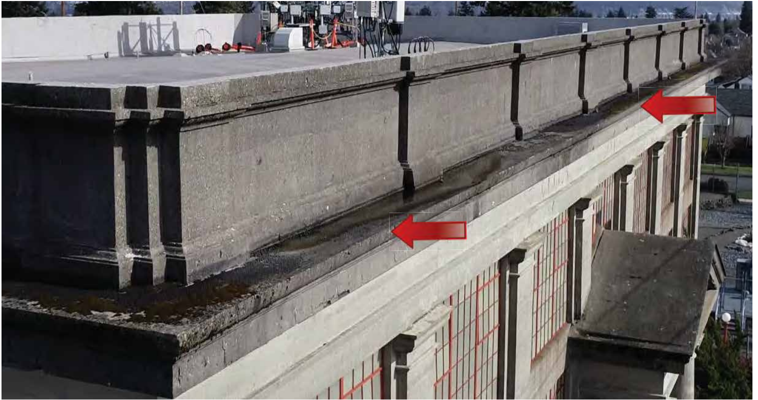
Organic soiling (algae, moss, etc.) and water collection observed on the cornice on the south elevation. 200224 CoT CAS EL-N DJI_00282.JPG
