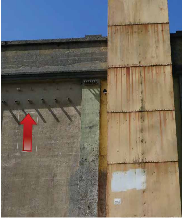
Observed steel eye bolts, pulleys, and severed tubes embedded into the concrete on the south elevation. The pipes embedded in the concrete appear not to be adequately sealed, allowing water infiltration into the wall. Image by Richaven Architecture and Preservation. 220620 CoT CAS EL-S P1000671.JPG
