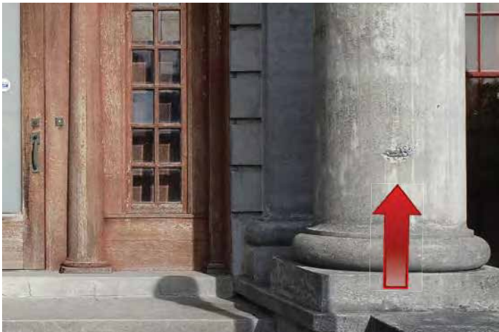
Damage to a column on the south elevation. Image by Richaven Architecture and Preservation. 200224 CoT CAS EL-S DJI_0027
