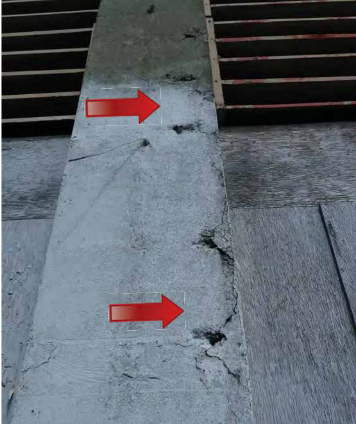
Severe spalling and cracking on a pilaster on the west elevation. Image by Richaven Architecture and Preservation. 220620 CoT CAS EL-E P1000678.JPG
