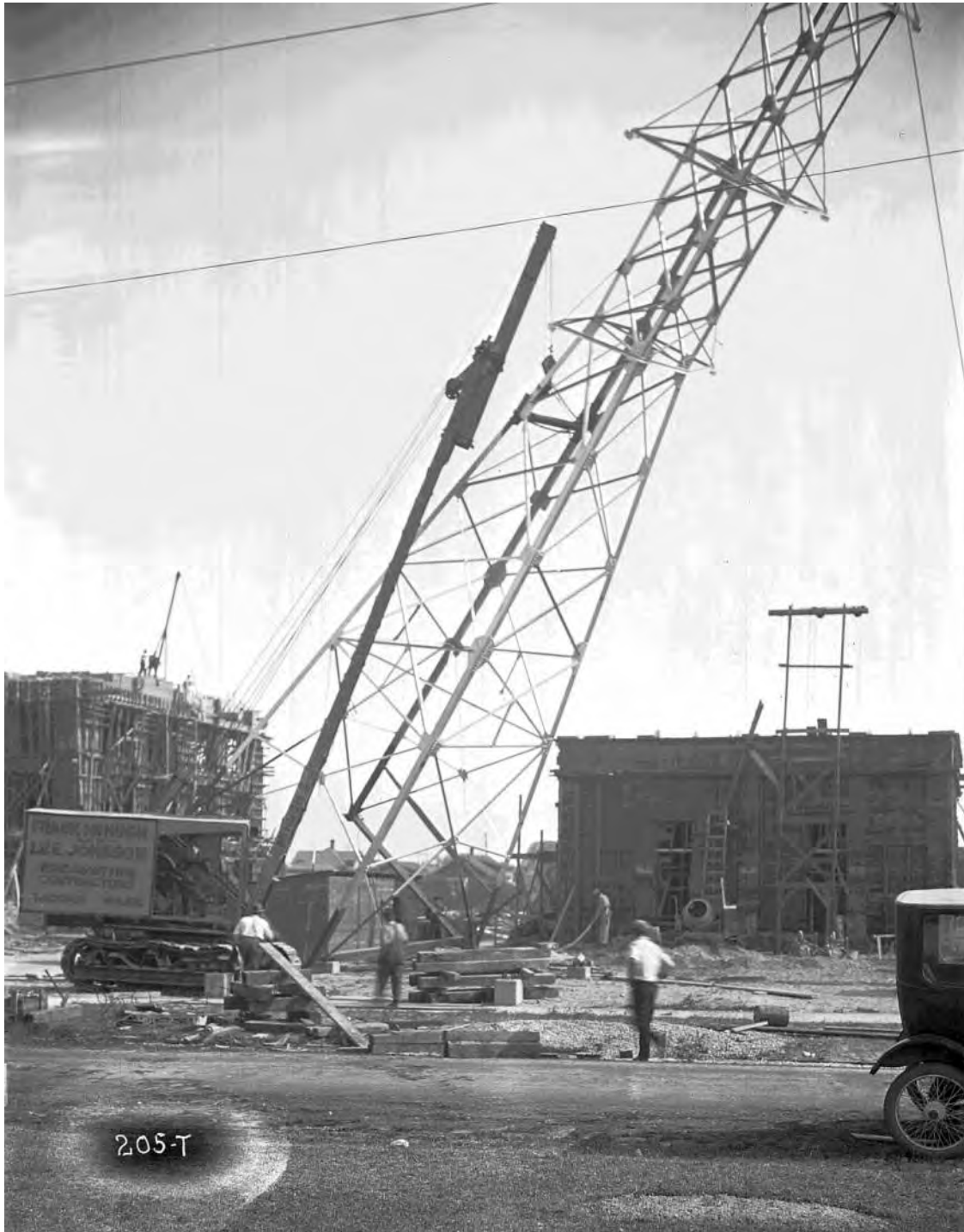
Figure 4. Steel lattice tower, constructed adjacent to the Adams St. Substation, view south, 1925. Courtesy of Tacoma Power.
