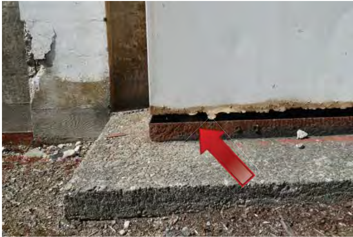
Richaven observed severe corrosion on the base of the steel ventilation stack on the south elevation. Image by Richaven Architecture and Preservation. 220620 CoT CAS EL-S P1000670.JPG
