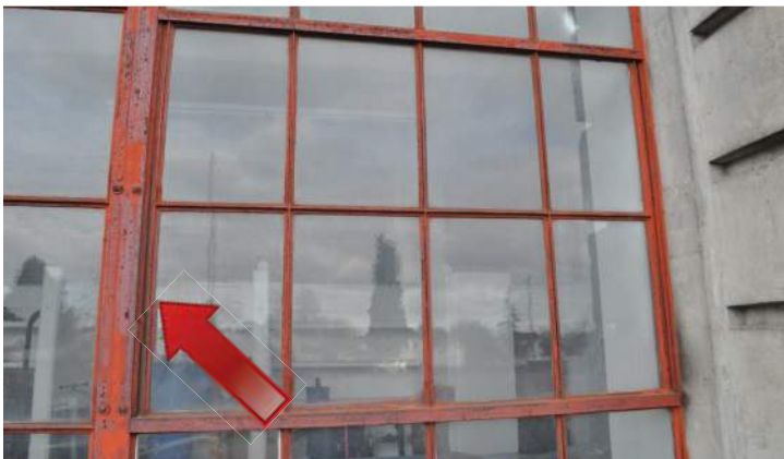
Operable sash-center-pivot exhibits corrosion and coating failure. Image by Richaven Architecture and Preservation. 200224 CoT CAS EL-N DSC_0176.JPG
