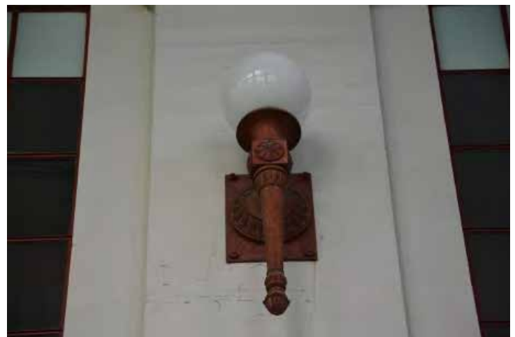
Cast iron decorative light fixture exhibiting corrosion. Image by Otak. 200224 CoT CAS INT DSC_0970.JPG
