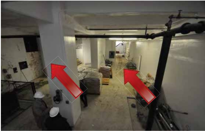
Paint failure on walls and soiling on the floor in the basement. Image by Otak. 200224 CoT CAS EL-INT DSC_0124.JPG
