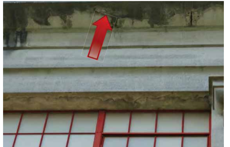
Build-up of airborne pollutants that have adhered and stained the concrete under the cornice on the south elevation. Efflorescence is also observed. Image by Richaven Architecture and Preservation. 220620 CoT CAS EL-W P1000666.JPG
