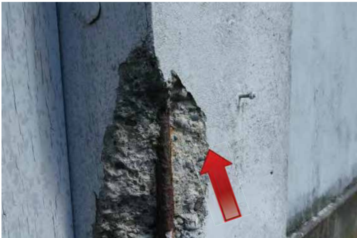
Spalling and exposed reinforcing steel immediately under cracks shown in the photo above. Image by Richaven Architecture and Preservation. 220620 CoT CAS EL-S P1000677.JPG
