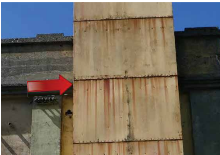
The panels that form the steel ventilation stack are severely corroded. Image by Richaven Architecture and Preservation. 220620 CoT CAS EL-S P1000671.JPG
