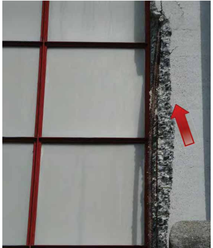
Severe spalling and separation from the substrate around a window on the west elevation. Image by Richaven Architecture and Preservation. 220620 CoT CAS EL-W P1000647.JPG
