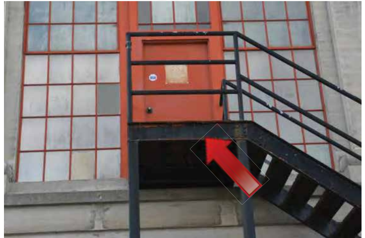
Door and stairwell on the second floor of the east elevation. Image by Otak. 200224 CoT CAS EL-E DSC_1039.JPG
