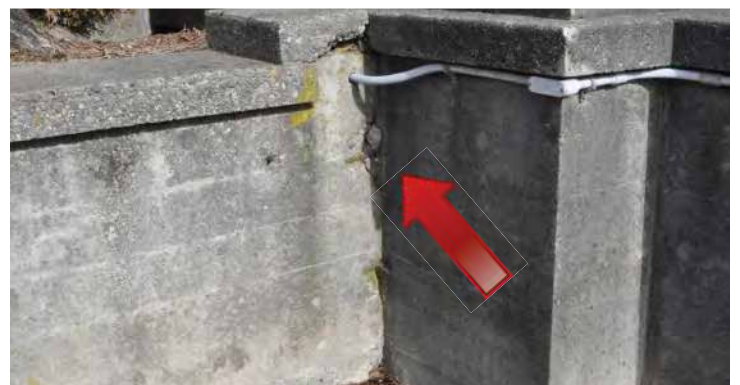
The foundation on the right side of the stairway has severe spalling, cracking, and organic soiling. Image by Richaven Architecture and Preservation. 200224 CoT CAS EL-S DSC_0014
