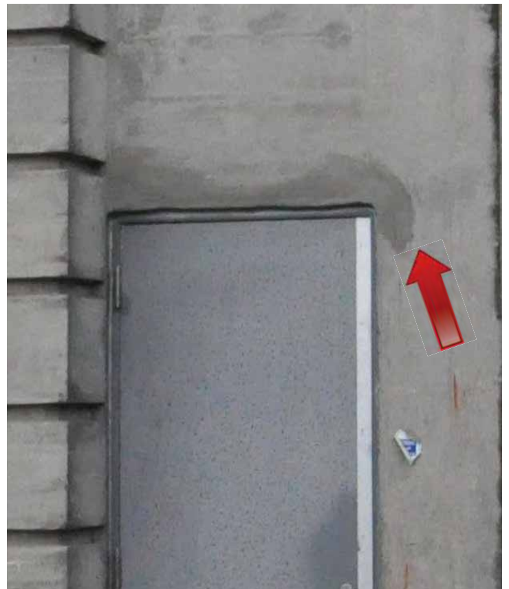
Cementitious repair above the door on the north elevation. Image by Richaven Architecture and Preservation. Image by Richaven Architecture and Preservation. 200224 CoT CAS EL-N DSC_0189.JPG
