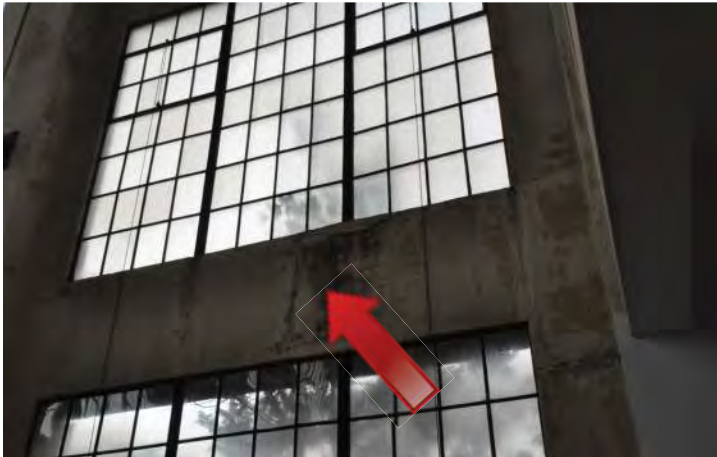
Soiling under the window appears to be mold and signs of water infiltration. Image by Otak. 200224 CoT CAS EL-INT DSC_0070.JPG
