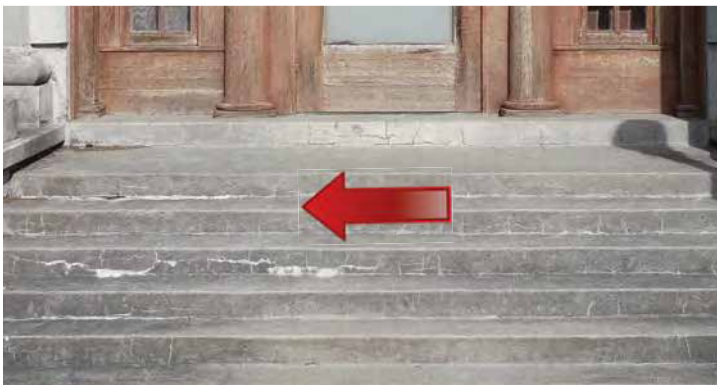
The stairway on the south elevation has severe spalling, cracking and soiling. Image by Richaven Architecture and Preservation. 200224 CoT CAS EL-S DJI_0027
