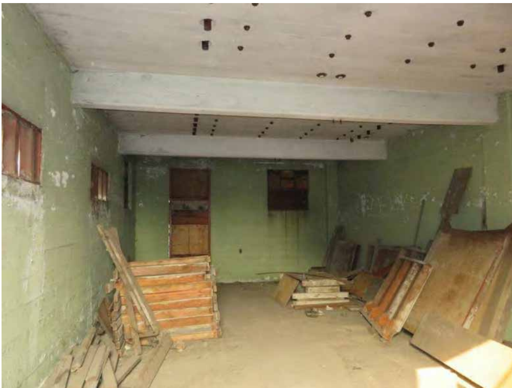
Photo 9 of 13. WA_PierceCounty_AdamsSt.Substation_0009. Adams St. Substation, interior, regulator room, lower level, view west.
