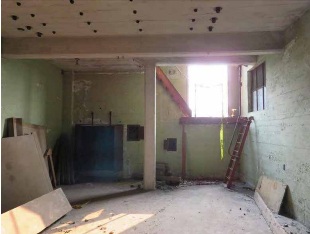
Photo 8 of 13. WA_PierceCounty_AdamsSt.Substation_0008. Adams St. Substation, interior, regulator room, lower level, view east.
