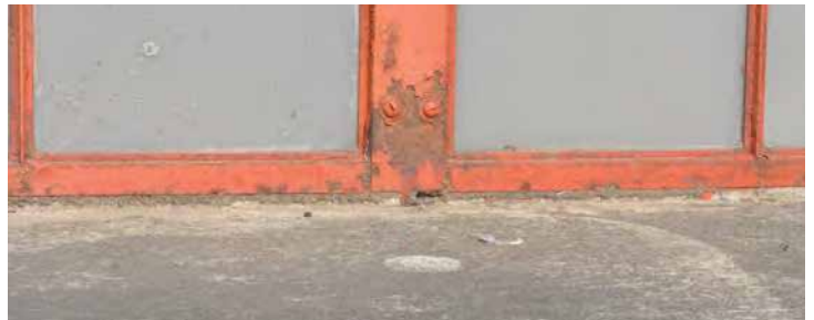
Most of the steel window frames on all elevations exhibit corrosion. Image by Richaven Architecture and Preservation. 200224 CoT CAS EL-W DSC_0020.JPG
