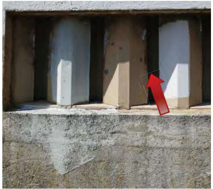
Vent on the south elevation with corrosion on the edges. Areas in white were painted to cover graffiti. Image by Richaven Architecture and Preservation. P000673.JPG.
