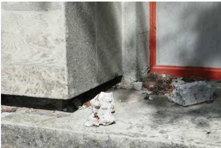
Failed concrete at one of the ground level window bays on the west elevation. Image by Richaven Architecture and Preservation. 220620 CoT CAS EL-W P1000660.JPG
