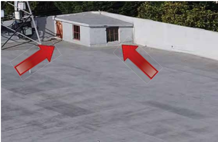
The door for roof access is badly corroded, and windows are starting to deteriorate. 200224 CoT CAS EL-S DJI_0037
