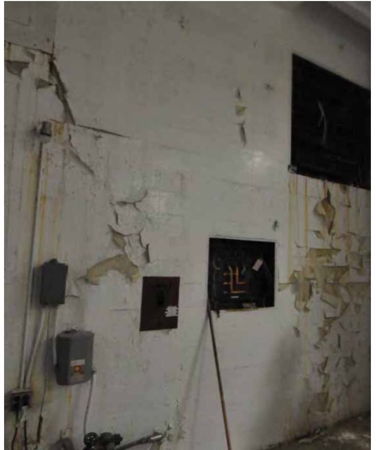
The location above shows concrete wall with the coating failing and peeling. Image by Otak. 200224 CoT CAS EL-INT DSC_0126.JPG.
