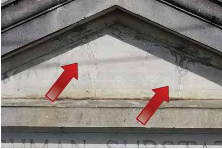
Spalling and efflorescence on the frieze. Image by Richaven Architecture and Preservation. 200224 CoT CAS EL-S DJI_00221.PNG
