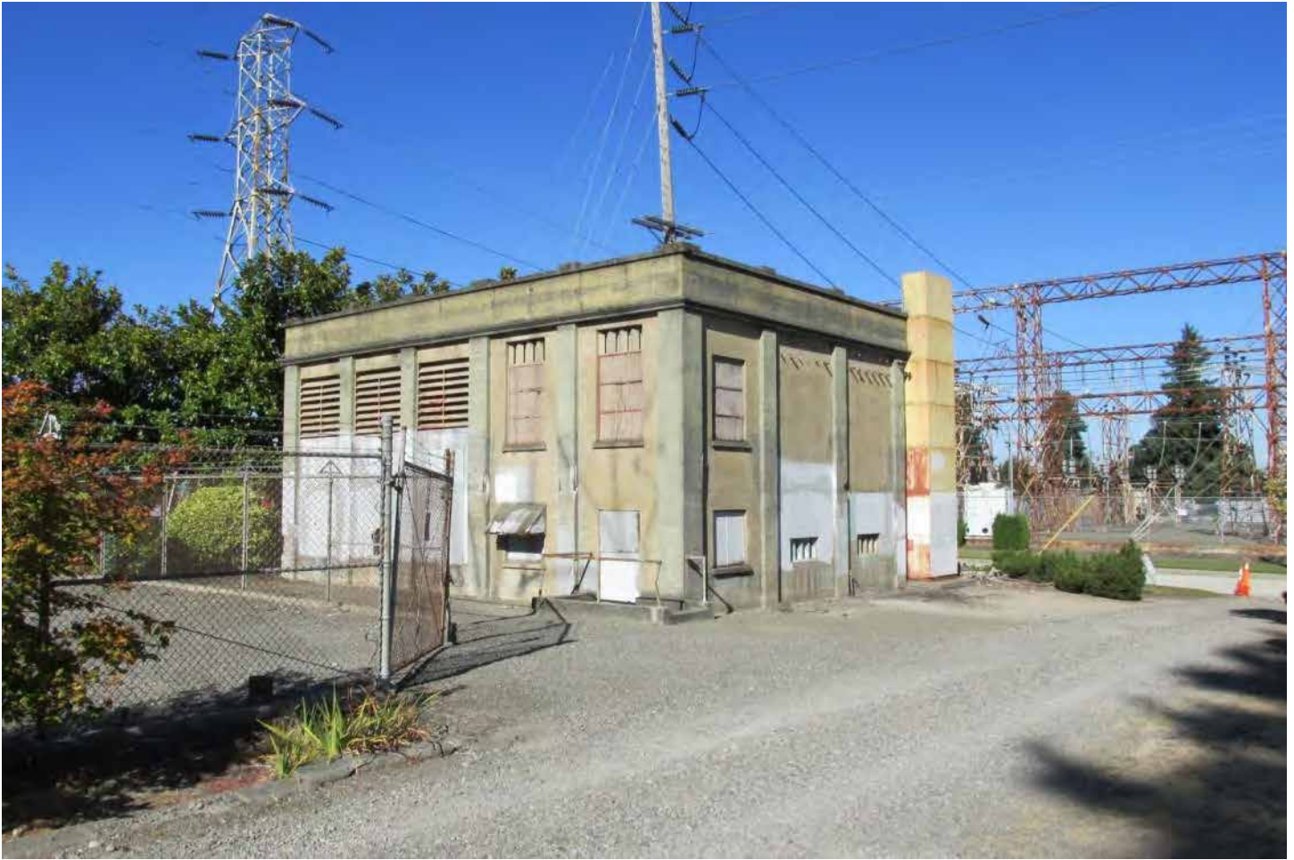
Figure 23 Adam Street Substation, with tower 1 in background, view northeast
