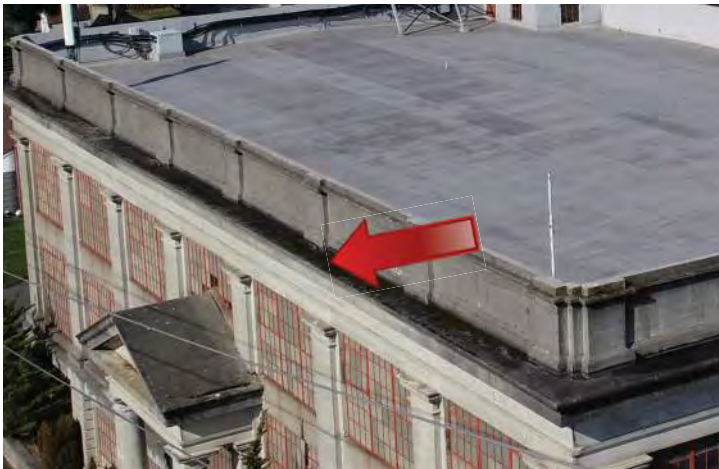
Algae growth on the cornice on the south elevation indicates that water is collecting. Image by Richaven Architecture and Preservation. 200224 CoT CAS EL-S DJI_0037.JPG
