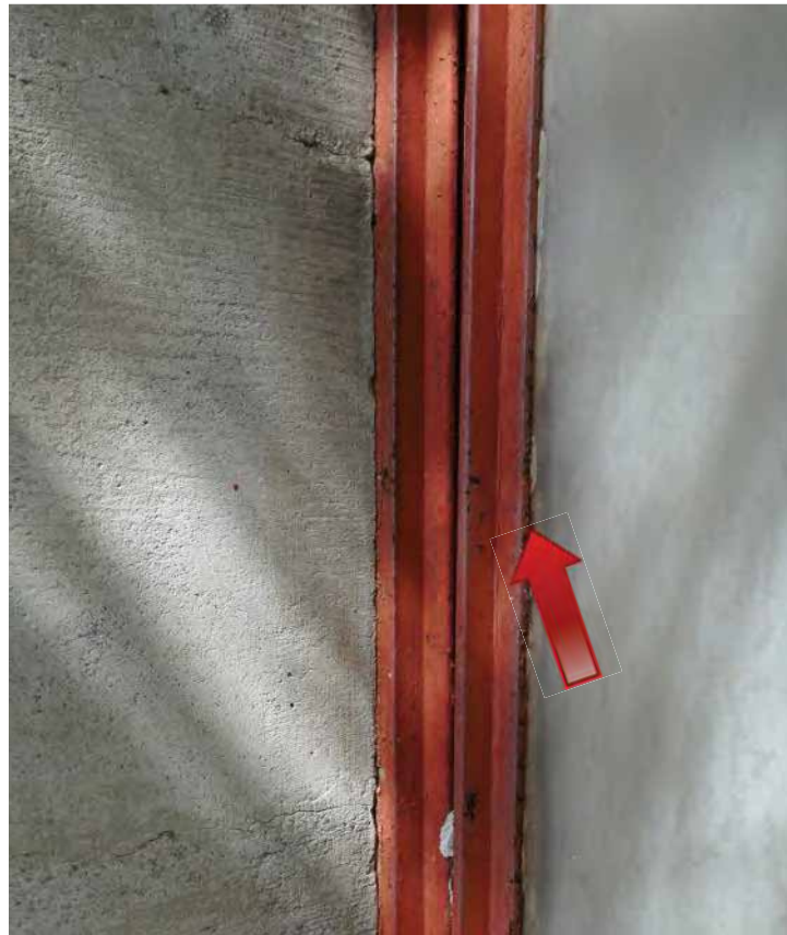
Detail of the cast-in-place steel window frame exhibits delamination, corrosion, and missing glazing compound. Image by Richaven Architecture and Preservation. 220620 CoT CAS EL-W P1000664.JPG
