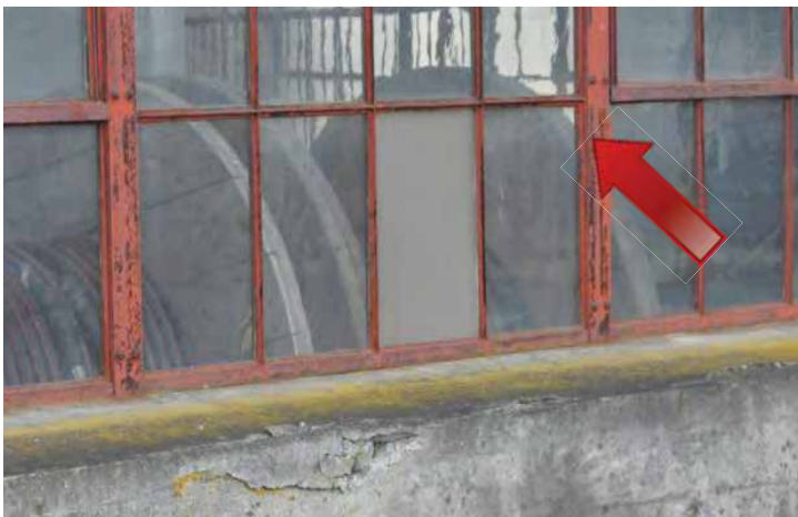
Mullions and muntins on all elevations exhibit corrosion and coating failure. Image by Otak. 200224 CoT CAS EL-N DSC_0184.JPG
