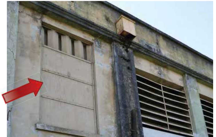
Missing steel windows and vents have been covered with plywood boards. Image by Richaven Architecture and Preservation. 220620 CoT CAS EL-E P1000691.JPG.
