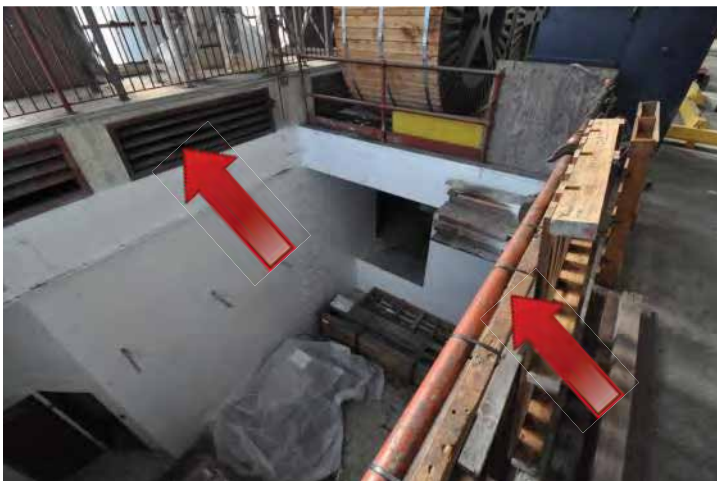
Visible soiling, corrosion, and paint failure over the vents and railings. Image by Otak. 200224 CoT CAS EL-INT DSC_0051.JPG
