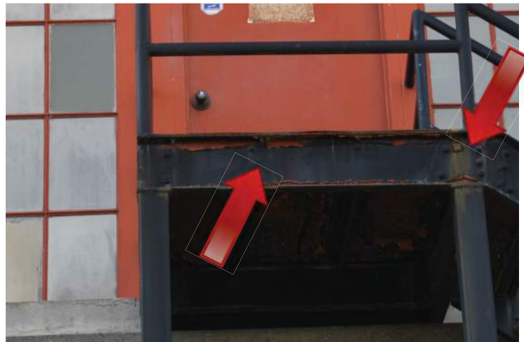
There is visible paint failure on the structure and signs of corrosion. Image by Otak. 200224 CoT CAS EL-E DSC_1039.JPG
