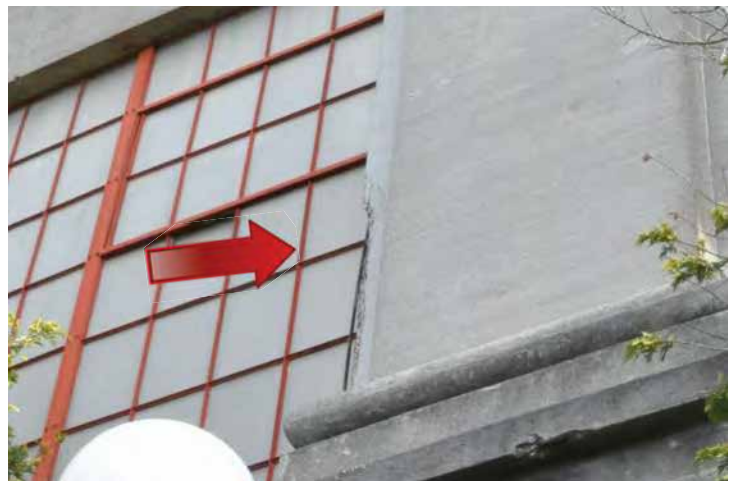
Severe separation from the substrate on the left edge of a pilaster on the west elevation. Image by Richaven Architecture and Preservation. 200224 CoT CAS EL-W DSC_0036.JPG
