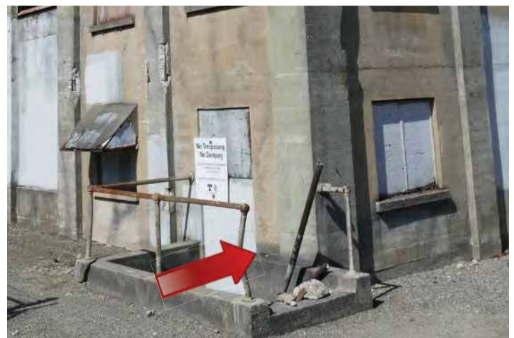
Pipe railings around the concrete stairway on the west elevation have failed. Image by Richaven Architecture and Preservation. 220620 CoT CAS EL-S-W P1000688.JPG
