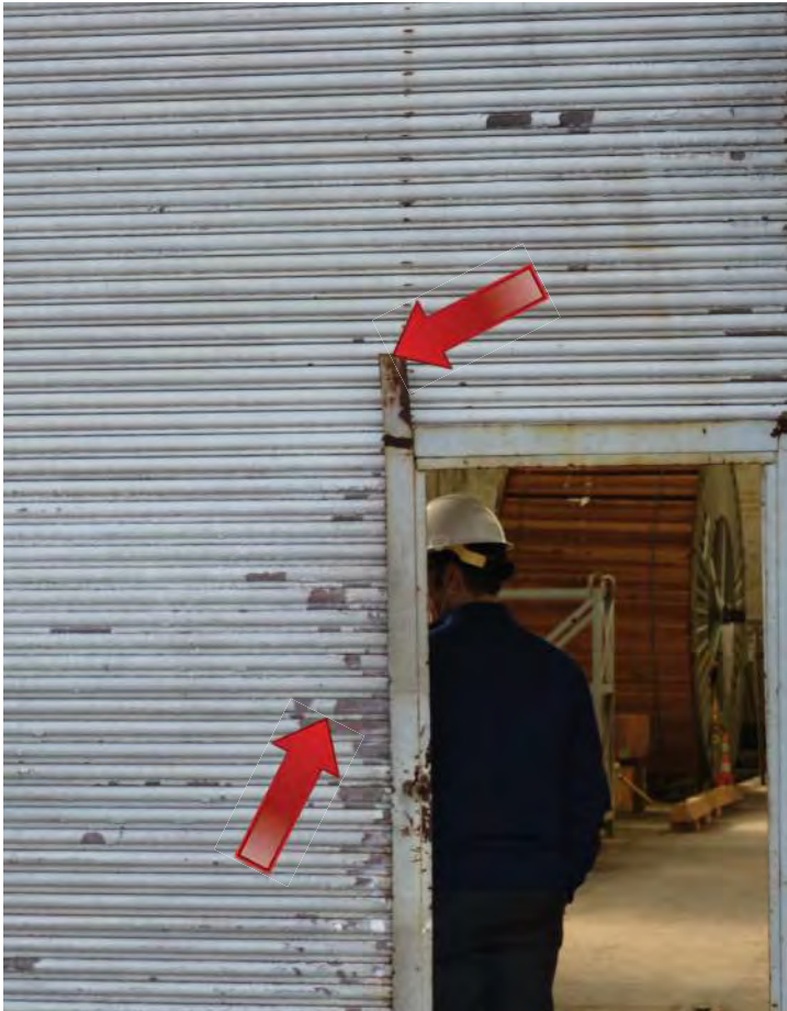
Richaven observed paint failure on the surface of the roll-up door on the north elevation, and corrosion around the steel frame door insert. Image by Otak. 200224 CoT CAS EL-E DSC_1056.JPG
