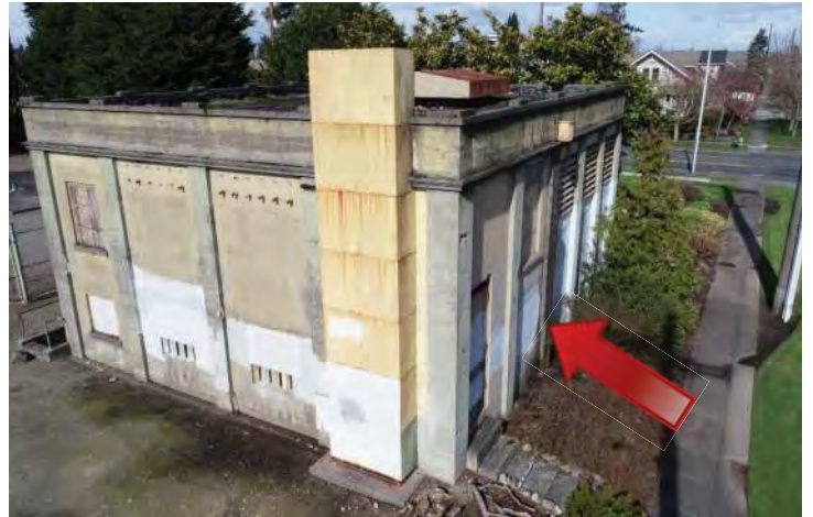
White paint used to cover graffiti. Image by Richaven Architecture and Preservation. 200224 CoT CAS EL-S-E DJI_0073.JPG
