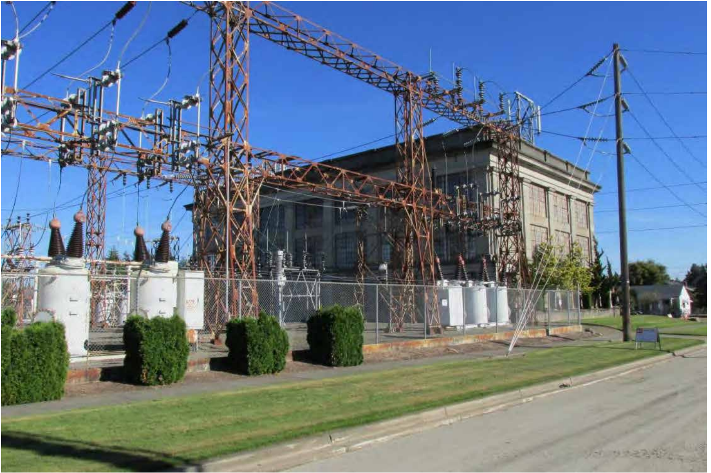
Figure 19 Cushman Substation view southeast
