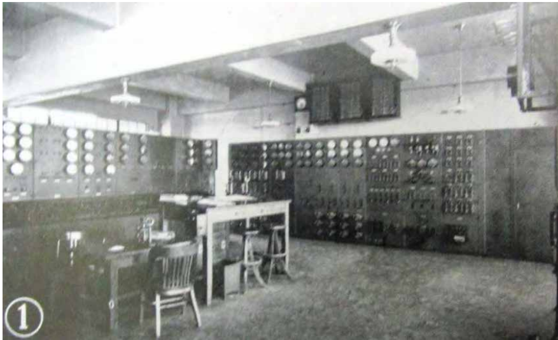
Figure 9 Cushman Substation Control Room ca. 1929, Image courtesy of Tacoma Public Library
