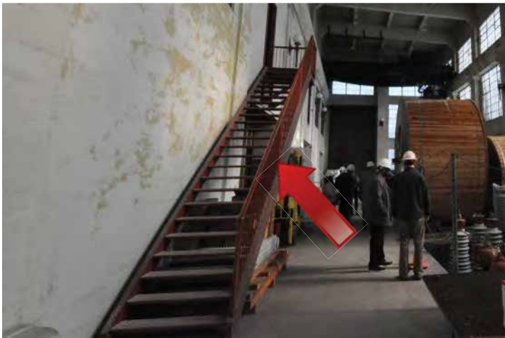
Dust / dirt soiling was observed on the stairwell. Image by Otak. 200224 CoT CAS EL-INT DSC_0065.JPG
