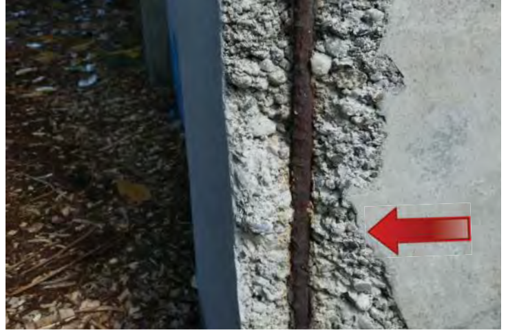
Failed concrete with exposed reinforcing steel on the left corner of a pilaster on the south elevation. Image by Richaven Architecture and Preservation. 220620 CoT CAS EL-S P1000675.JPG
