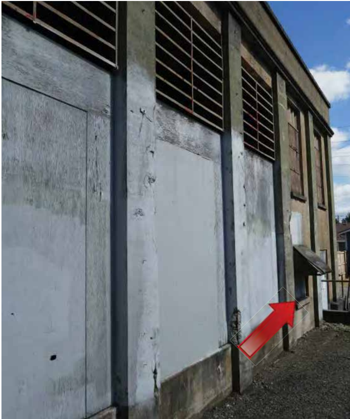
Metal louvers on the west elevation and a missing window covered with plywood boards. Image by Richaven Architecture and Preservation 06/20/22, 220620 CoT CAS EL-W P1000674.JPG
