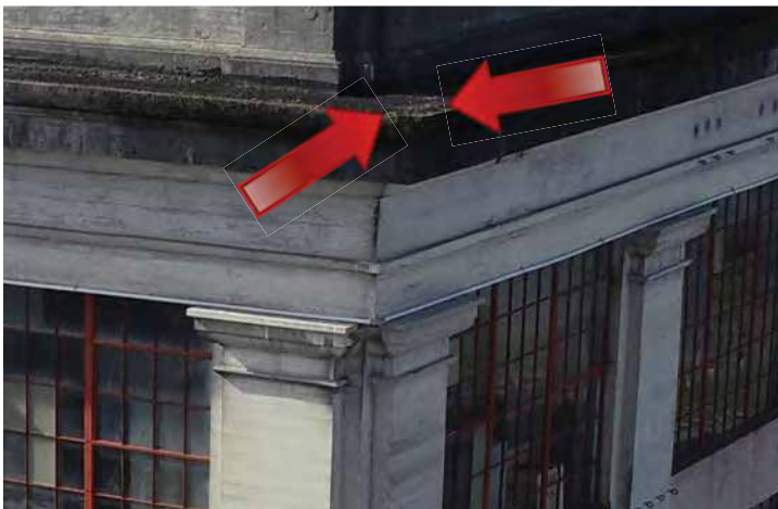
Water proofing on top of cornice, on the east corner of the south elevation appears to be failing. Image by Richaven Architecture and Preservation. 200224 CoT CAS EL-S-W DJI_00036.jpg
