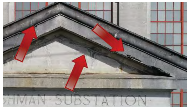
Pediment above the main entrance on the south elevation shows severe spalling, efflorescence, and atmospheric soiling. Image by Richaven Architecture and Preservation. 200224 CoT CAS EL-S DJI_00221.PNG
