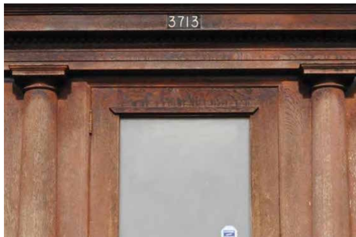
Door frame with a significant amount of fading and discoloration. Image by Richaven Architecture and Preservation. 200224 CoT CAS EL-S DSC_0011.JPG
