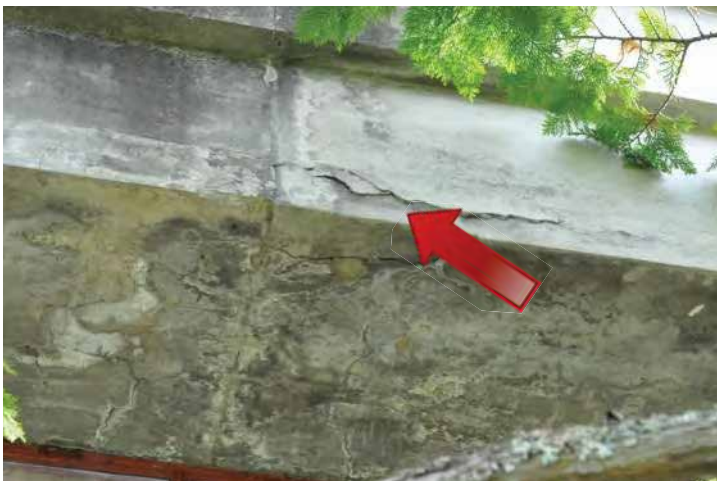
Cracking and delamination present above a window on the west elevation. Image by Richaven Architecture and Preservation. 200224 CoT CAS EL-W DSC_0035.JPG
