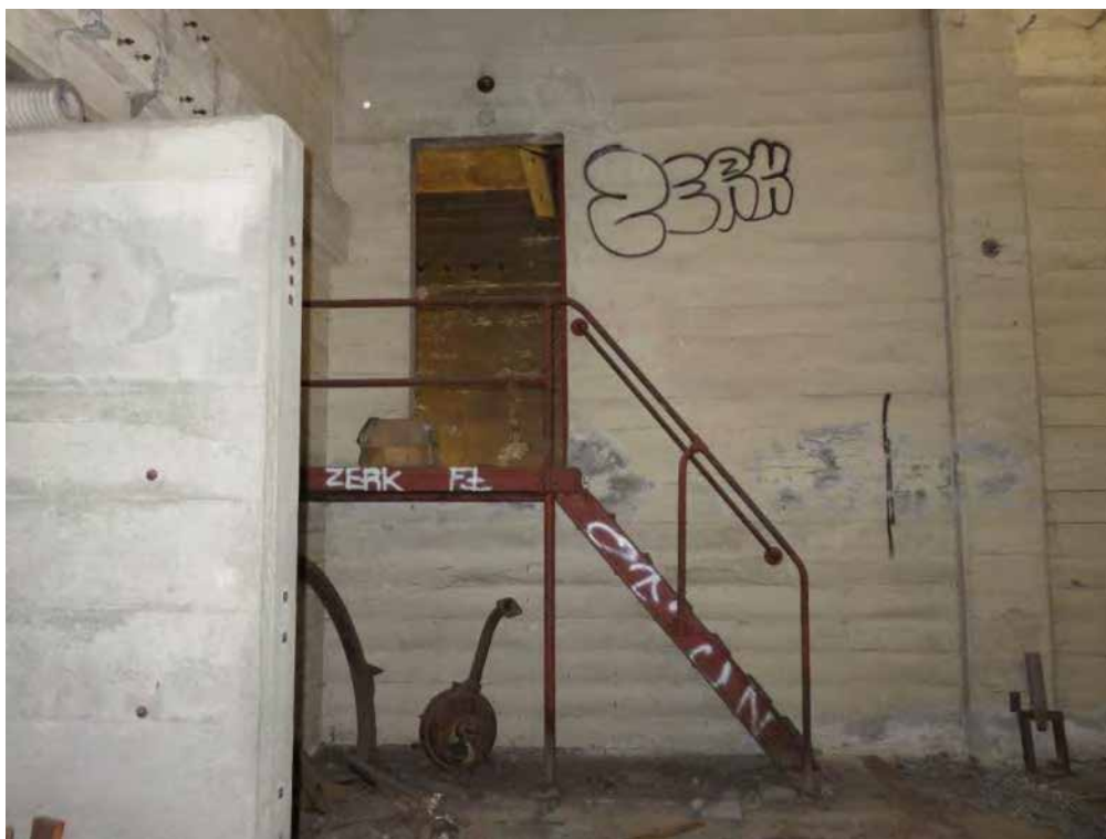
Photo 12 of 13. WA_PierceCounty_AdamsSt.Substation_0012. Adams St. Substation, interior, transformer room, view south.
