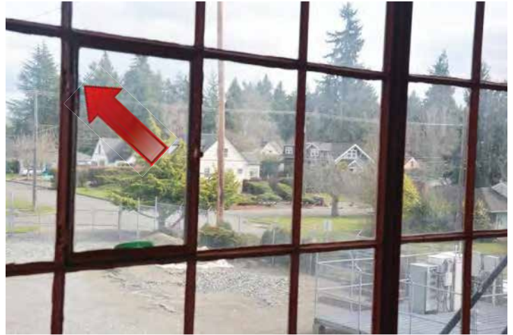
Badly corroded steel window frames and loss of glazing compound. Image by Otak. 200224 CoT CAS EL-INT DSC_10099.jpg
