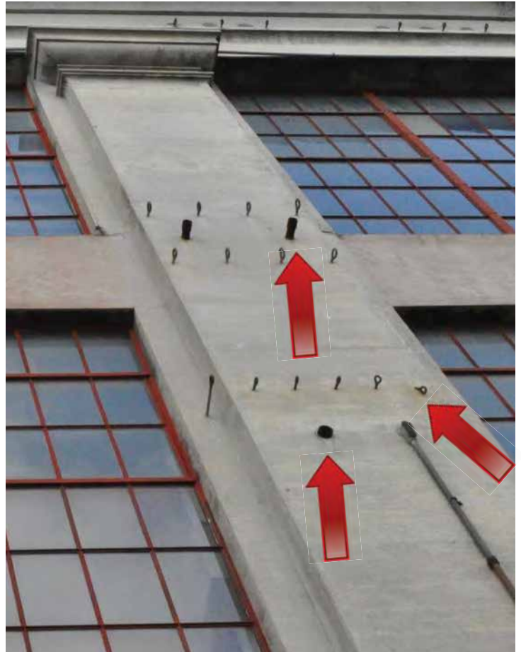
Observed steel eye bolts and several tubes embedded in the concrete on the east elevation. Image by Richaven Architecture and Preservation. 200224 CoT CAS EL-E DSC_0189.JPG
