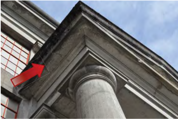
Efflorescence was observed under the pediment and entablature on the main entrance. Image by Richaven Architecture and Preservation. 200224 CoT CAS EL-S DSC_0016.JPG
